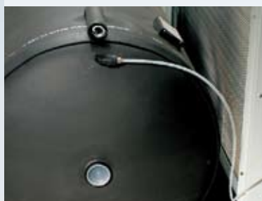
Large buffer tank.
