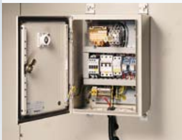
Integral independent electrical panel.
